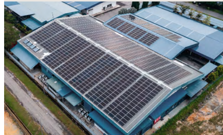
Solar panel on the roof of Micromechanics Malaysia.
